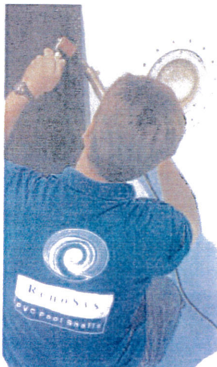
Hot air thermal fusion welding bonds the membrane to the pool surface, creating a permanent
